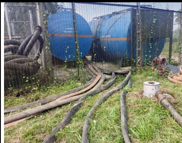
WATER HOLDING TANKS
