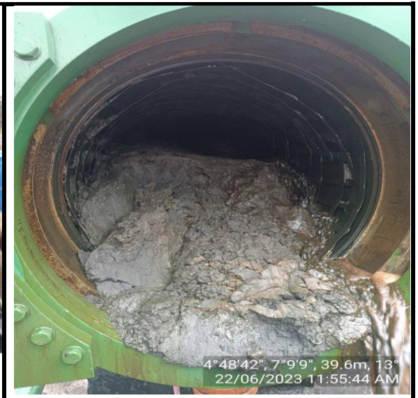
DEBRIS PUSHED OUT BY PIG
