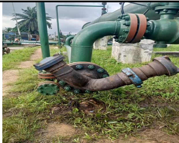
INSTALLED HOOK UP POINTS
