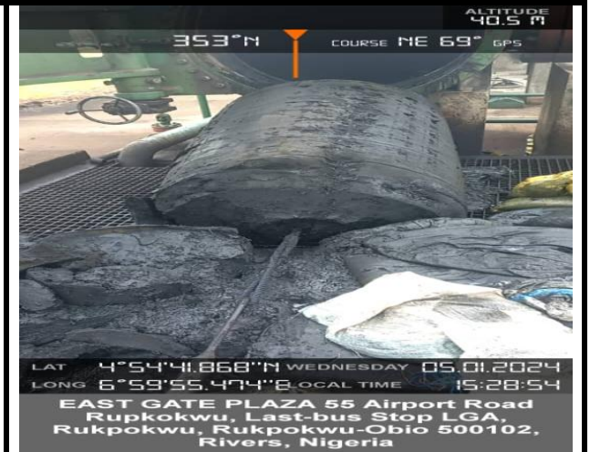
RECOVERED 36" MD FOAM PIG WITH DEBRIS
