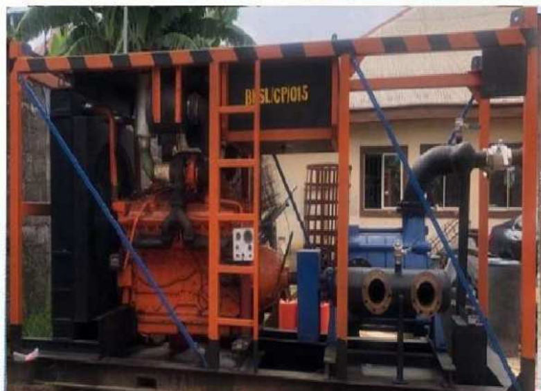
90BBLs/MIN @ 300Psi PIPELINE FLOW AUGMENTATION EQUIPMENT
