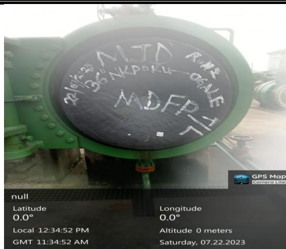
LOADED 36" MD FOAM FLUSHING PIG RUN 2
